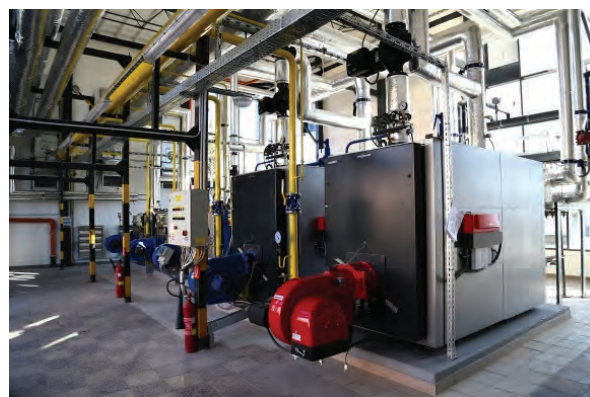
Fig. 6 - View to the reconstructed hot-water boiler house on natural gas
