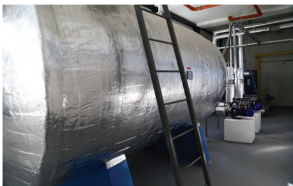
Fig. 4 – Lying accumulation and degassing tank with volume 10 \text{ m}^3
