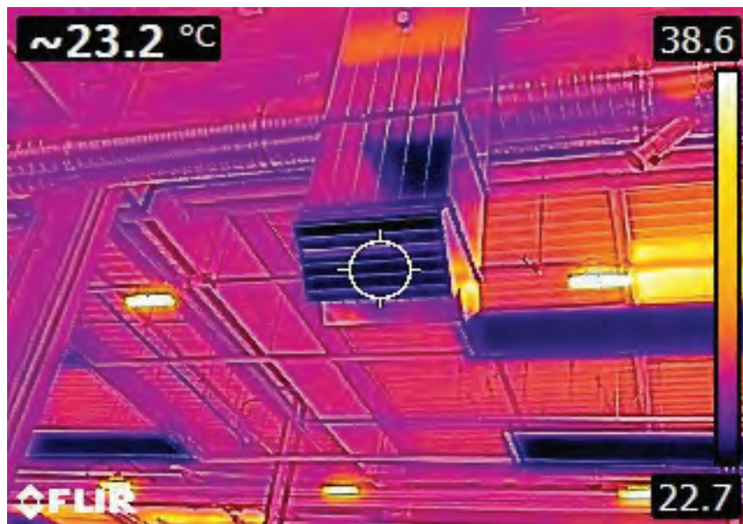
Fig. 6. Supply air temperature distribution at the outlet of the adiabatic cooler.
