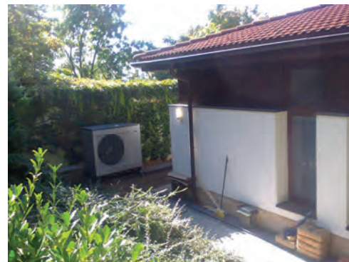
Fig. 1 Outdoor unit of Air/Water HP
