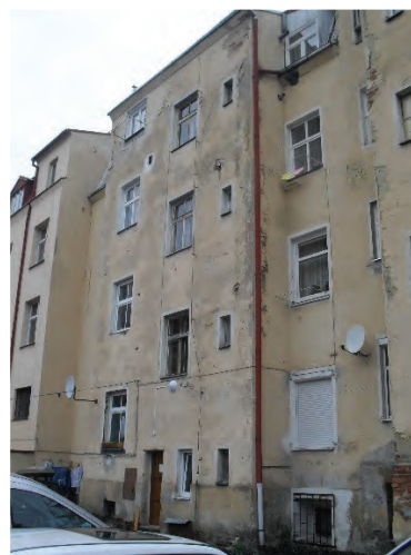
Figure 1b. Residential building with uninsulated part of the envelope [6]
