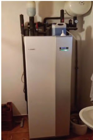
Fig. 4 Indoor unit of HP system
