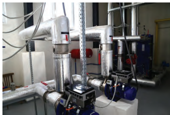
Fig. 5 – View on the plate heat exchangers HEX1 and HEX2, in foreground are circulating pumps
